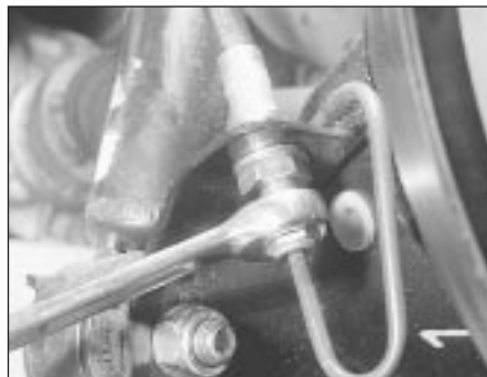
21.3 Undoing a rigid pipe union nut Flexible hose locknut is just above
